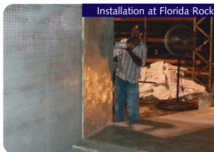
Installation at Florida Rock
